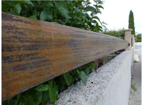
Vertical enclosure on a low wall without a guard rail, Teyran (France).
