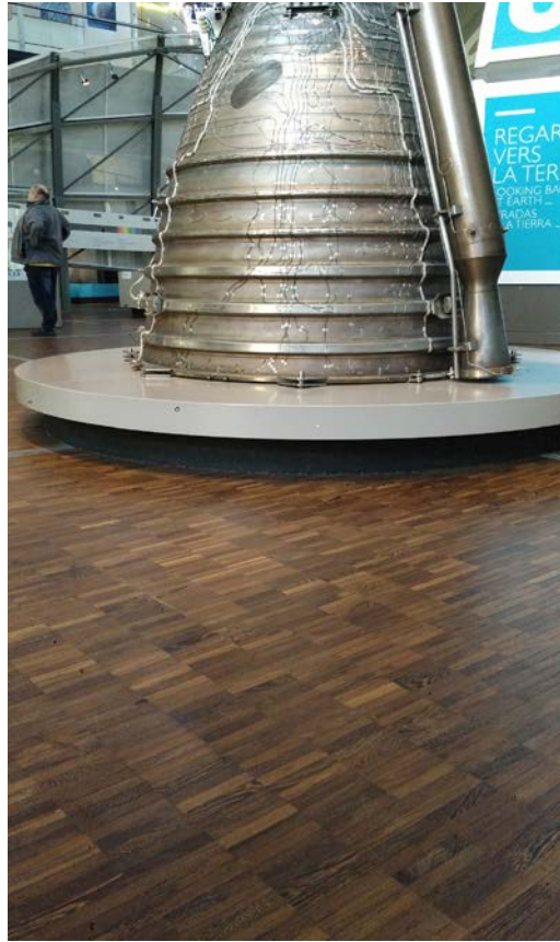
Parquet flooring of an exhibition gallery at Parc de la Villette – Paris (France).
