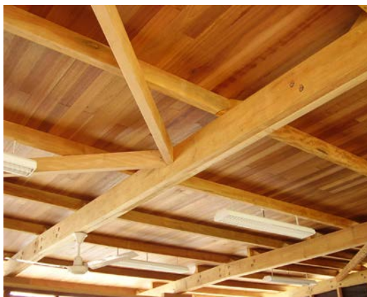
Basralocus sheathing on a ceiling frame in Mandioqueira, Gontran Damas secondary school, Cayenne (French Guiana).
