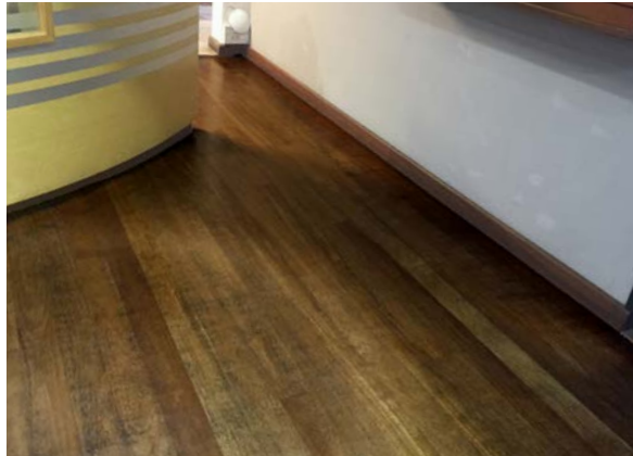
Floor at the offices of Fibres Industries Bois, Saint Paul, La Réunion (France).
